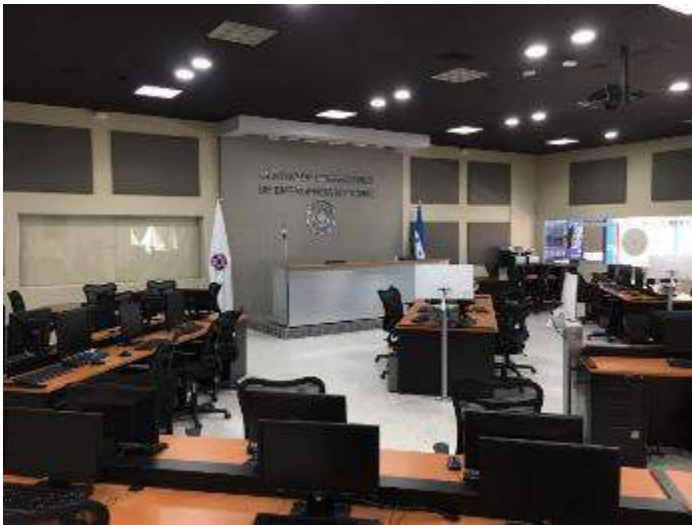
Figure 40. National EOC (COEN), Tegucigalpa, Honduras.
